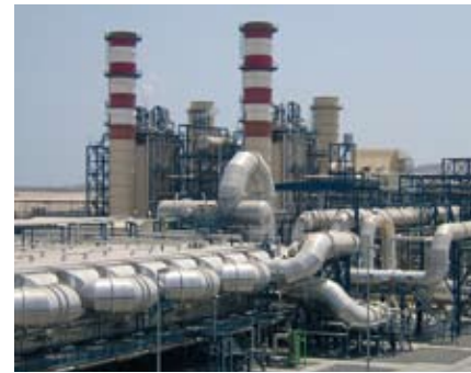
A thermal, multi-stage flash distillation (MSF) plant, in which successive condensation of evaporated brine generates energy for the next step.
