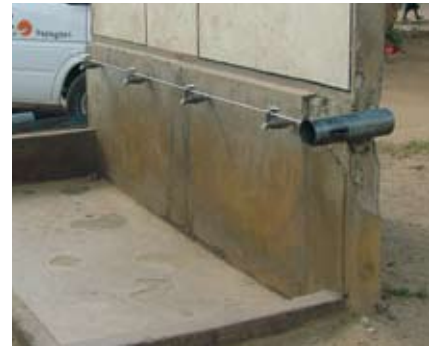
Water stand post for peri-urban area water supply, Lusaka, Zambia.
