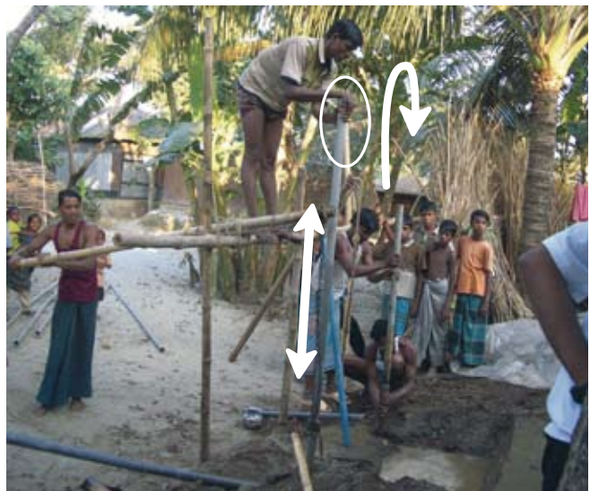
Figure 2. Hand percussion drilling for installation of the domestic tube wells by local drillers in Bangladesh. The block arrows indicate the flow of water during the washing process of drilling.
